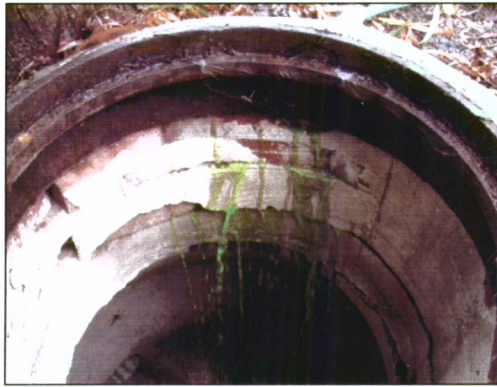
Dye from manhole defect
